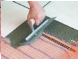
Comb thin-set mortar over the HeatWeave mats and lay tile on top.
