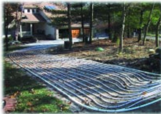
Snowmelt tubing installed in a residential driveway prior to pouring the concrete.
